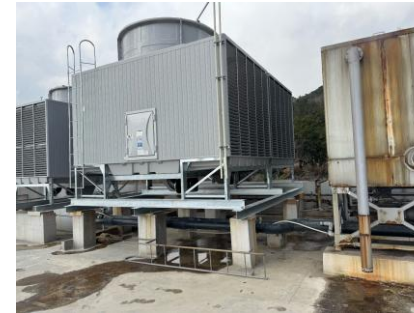
(An air conditioning system powered by geothermal steam naturally emitted on-site - Kirishima Kokusai Hotel)
